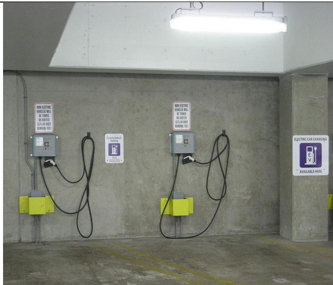
Wall-mounted charger: Note that electrical panels are protected by the yellow part. Signs indicated Electric Vehicle Charging Only.
