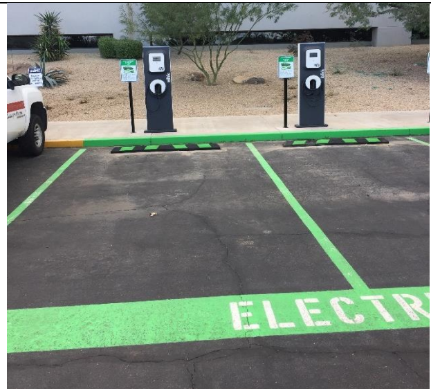
Pedestal-mount charger: Note the parking spaces are clearly marked with green paint and signs. The chargers are protected with a curb and curb stop. Bollards could be installed for additional protection.
